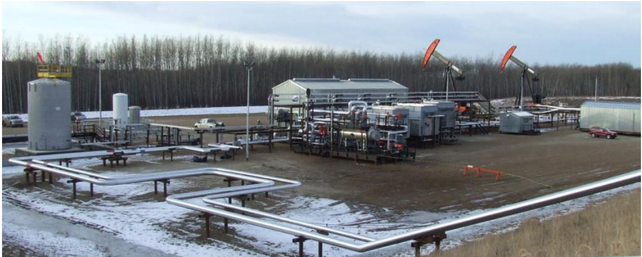
Figure 5 – T13 surface facilities.
