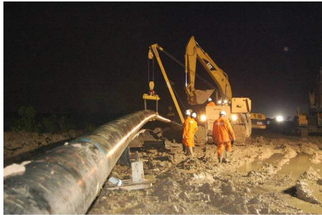
Picture of the Urucu/Manaus Gas Pipeline taken in December, 2006. [MostraTic, page 1]
