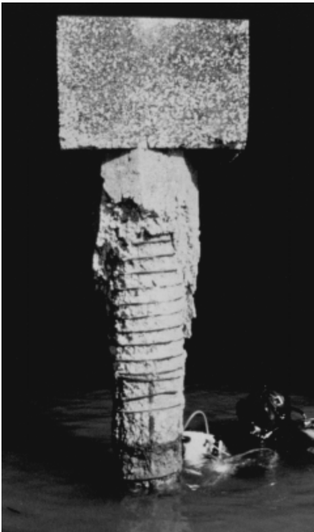
Fig. 1.2—Deteriorated piles in tidal and exposed zones. (Courtesy of I. Leon Glassgold.)
