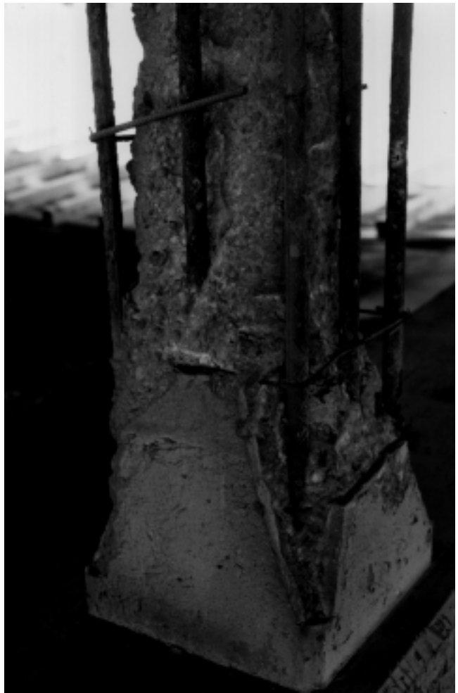
Fig. 1.3—Advanced deterioration, pile has been cleaned. (Courtesy of I. Leon Glassgold.)
