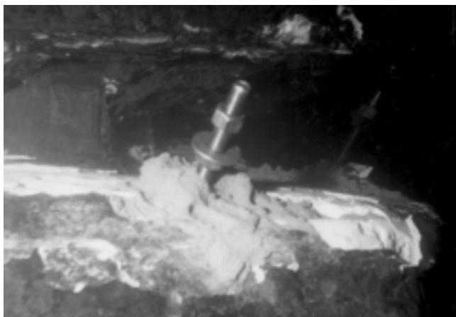
Fig. 6.1—Underwater view of hollow rock bolts grouted into existing construction. (Courtesy of M. Garlich.)
