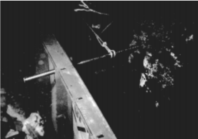
Fig. 5.1—“Symonds” forms in place underwater for pumped repair. (Courtesy of M. Garlich.)
