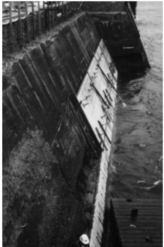
Fig. 5.2—Lower of three tiers of panels used to overlay the Troy Lock river wall were placed and infilled under partially submerged conditions. (Courtesy of J. McDonald.)
