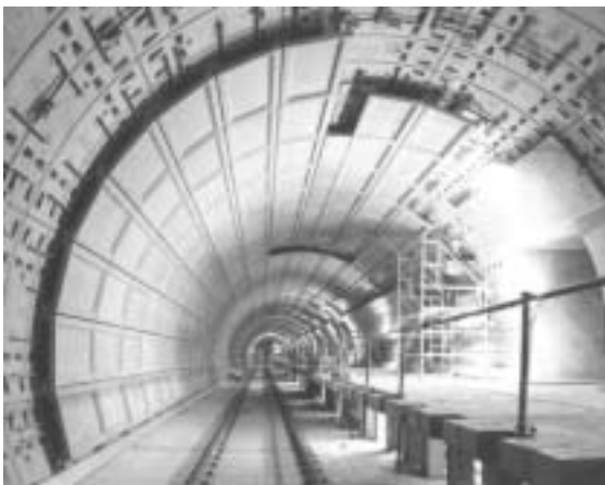
Fig. 5.10—Thin reinforced cementitious panels used as tunnel linings, Heathrow Express Railway Station, Heathrow Airport, London.
