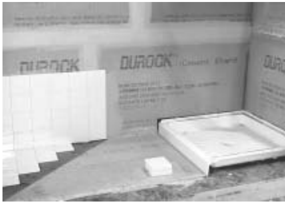
Figure 5.5—Mesh-reinforced cement board substrate for installation of ceramic tiles in wet areas (walls and floors) in buildings.
